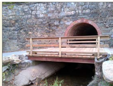
"Newly constructed bridge access to Fletcher's Cove built by U.S. Park Service personnel" (photo by Brian Hixon, provided by Steve LeBel)
